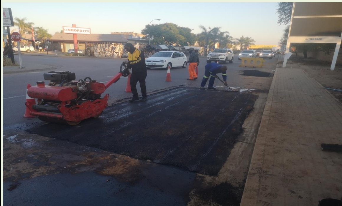
Damaged road with potholes
